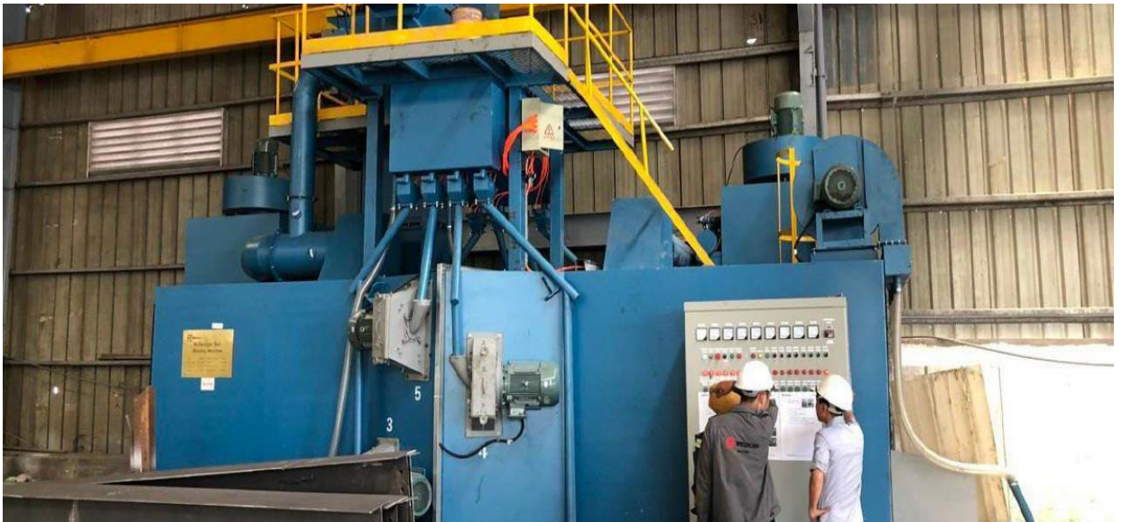
SHOT BLASTING LINE & PAINTING LINE
